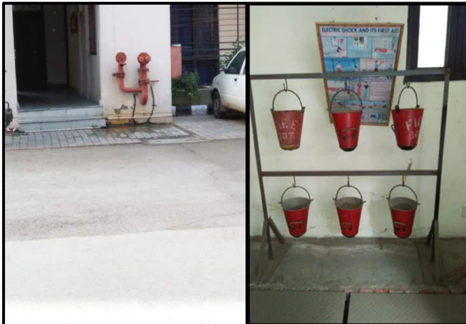
Fire Fighting Equipment
